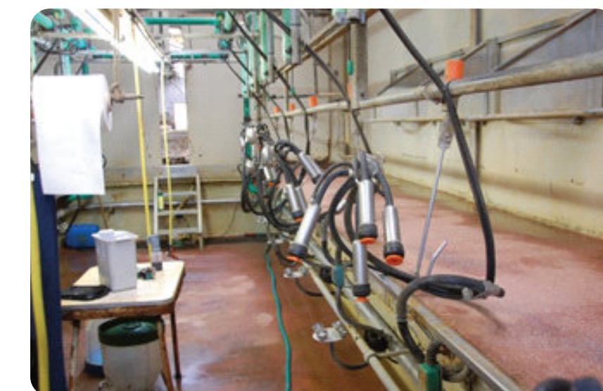
Milking parlor must be in 'dry test' during falloff test
